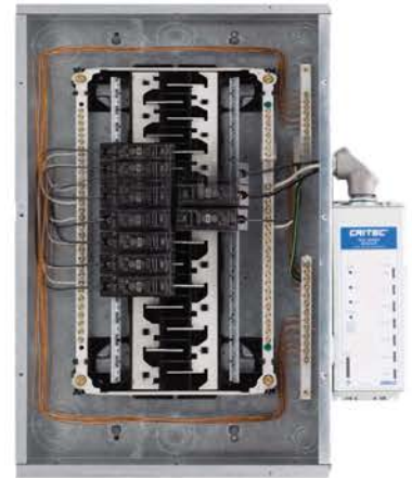
A Surge Suppression
